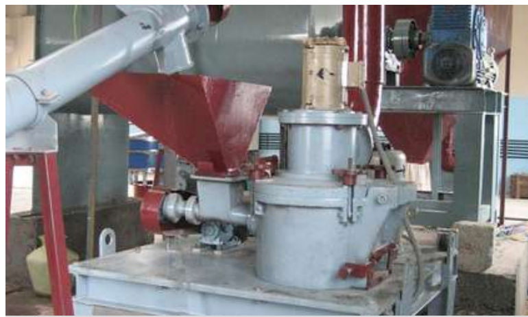
► Installation of DP® ACM-10 in South India for grinding of phenolic resin
