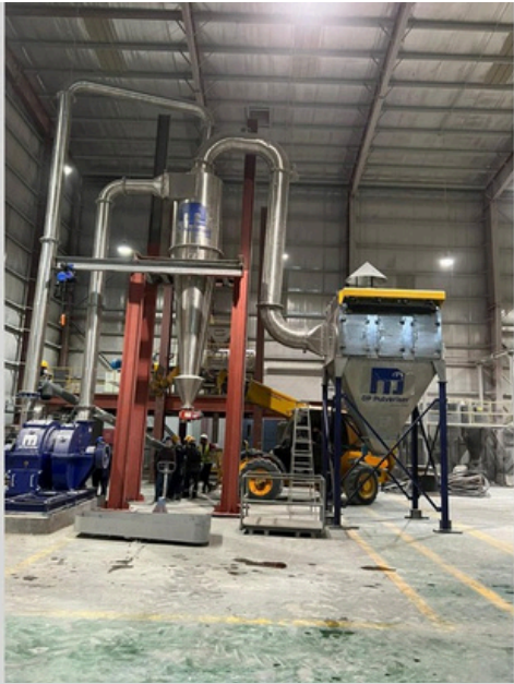
▶ DP® IP52 Impact Pulveriser for processing of Bentonite at Damman, Saudi Arabia
